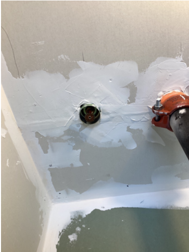
Building 5 missing plate
