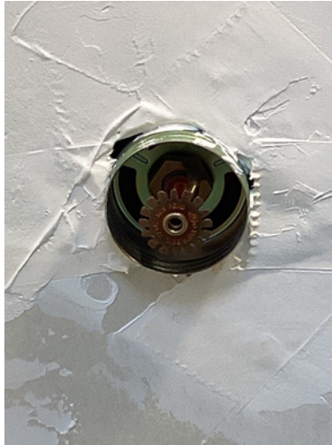
Building 5 missing plate
